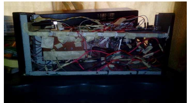
Figure 6: Completed ROEEMS circuitry
