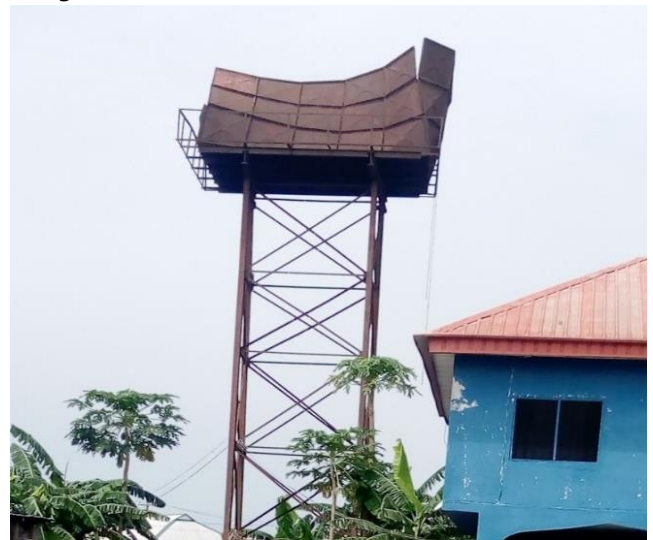
Figure 2: Elevated steel water stanchion.
