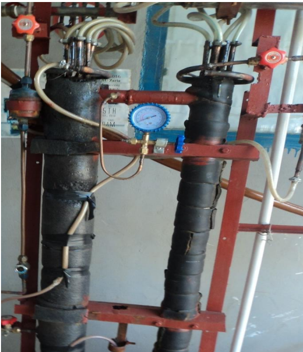
Figure 4: Close up view of Absorber and Evaporator
